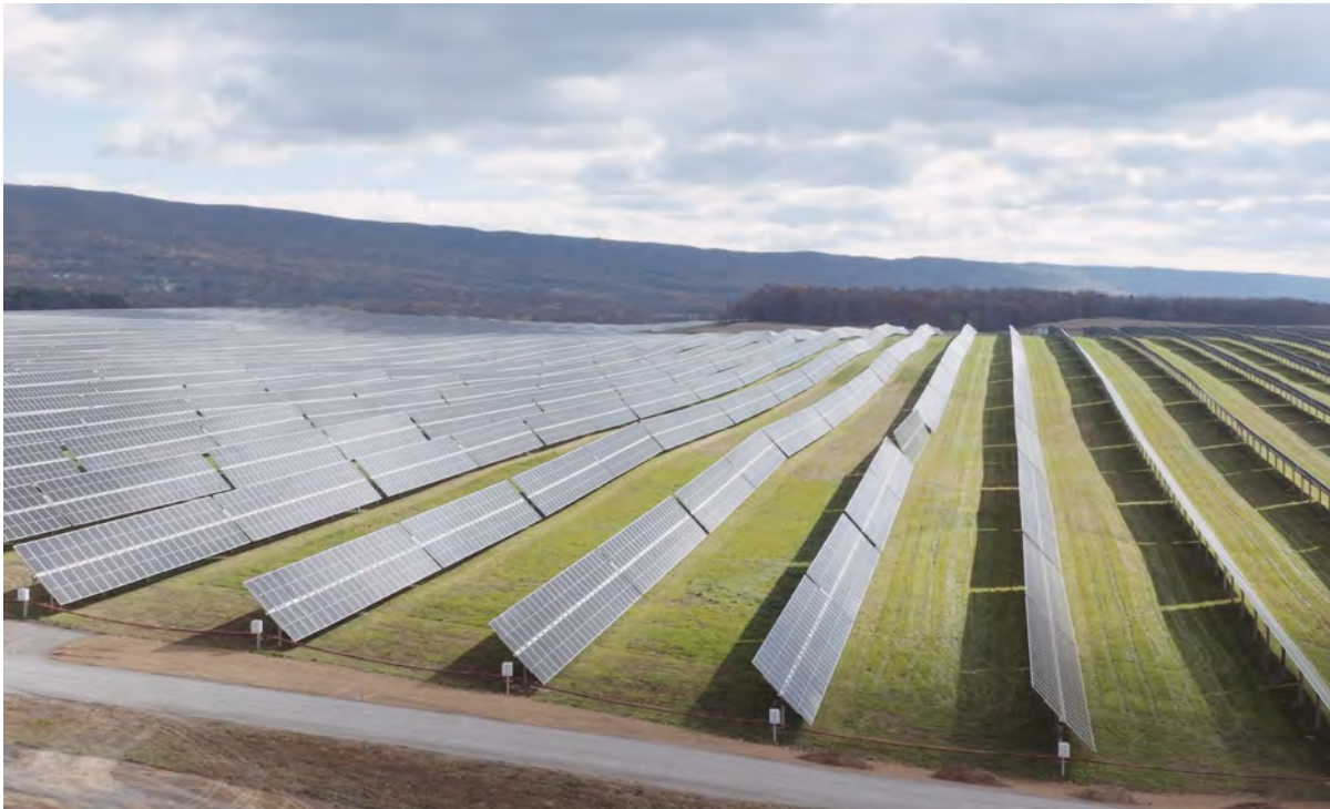
Penn’s Solar Power Purchase Agreement became operational in December 2023 when Great Cove 1 and 2 facilities were constructed in central Pennsylvania.
