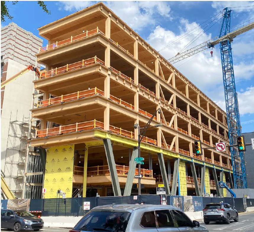
Amy Gutmann Hall, completed in 2024, is Philadelphia's tallest new mass timber building, with a cutting-edge system that significantly reduces the building's carbon footprint – by 52% relative to concrete, and 41% relative to steel.
